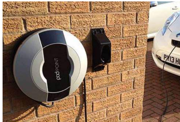
Figure 72: Home electric vehicles charging point
