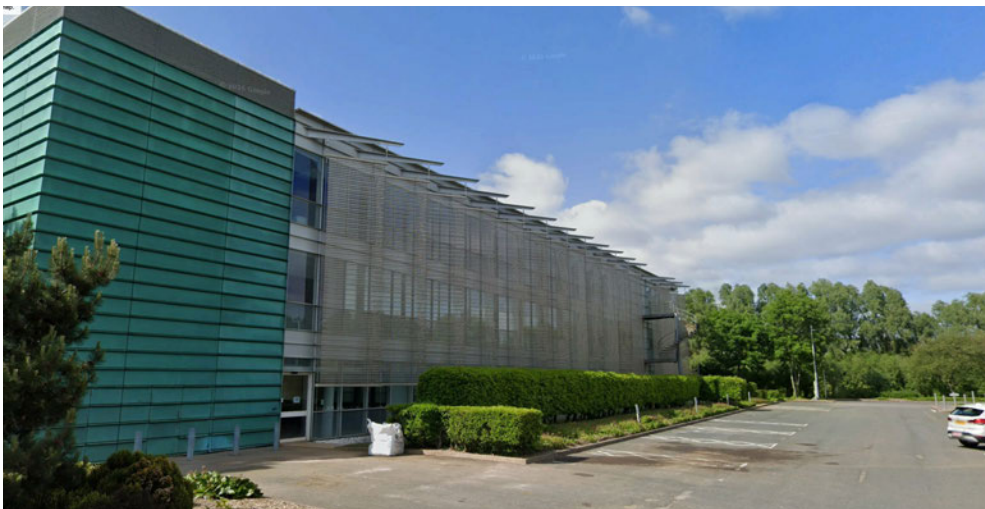
External solar shading, Green Park, Reading
