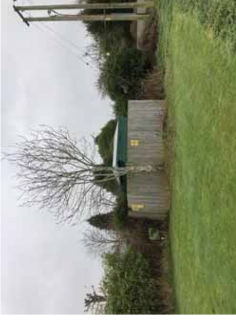
Photo 3: Substation in North-West
