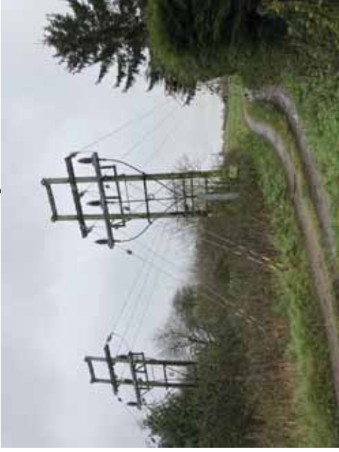
Photo 2: Overhead Electricity Lines in North-West
