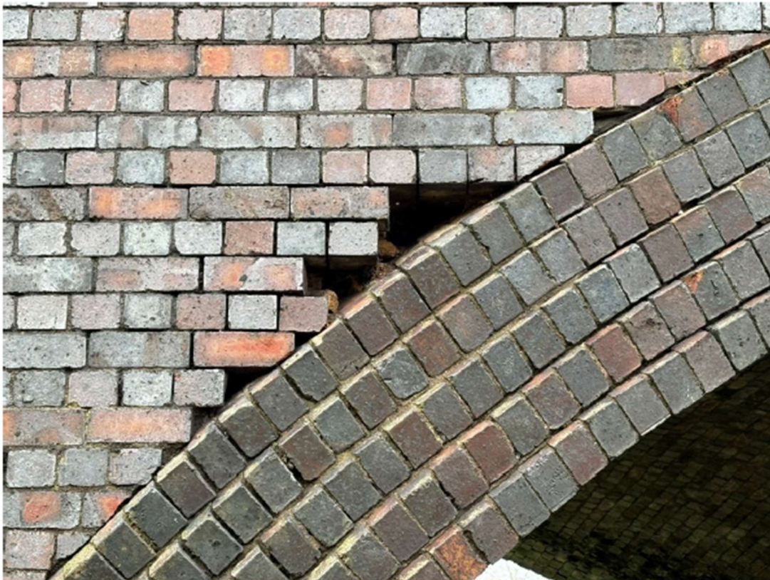
Photograph 62: Missing bricks on extrados and mortar in poor condition surrounding it
