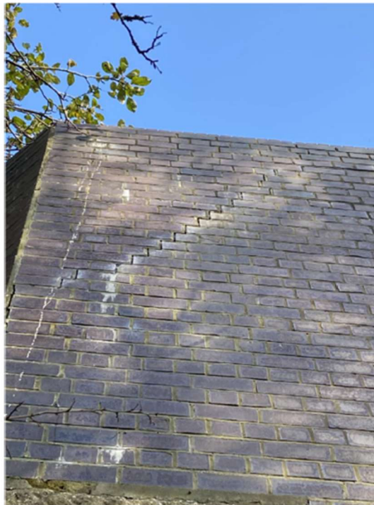
Figure 5.6: Significant stepped cracking with associated leaching found to the west end of the south wall
