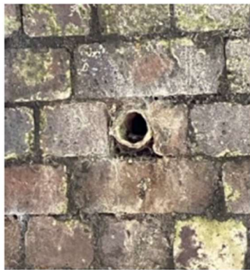
Figure 5.24: North span corroded drainage pipe
