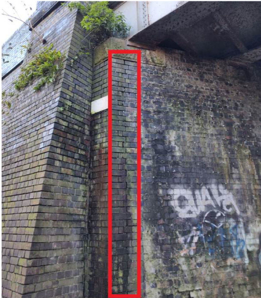
Figure 4-6 - Northeast abutment - full height cracking to masonry below padstone
