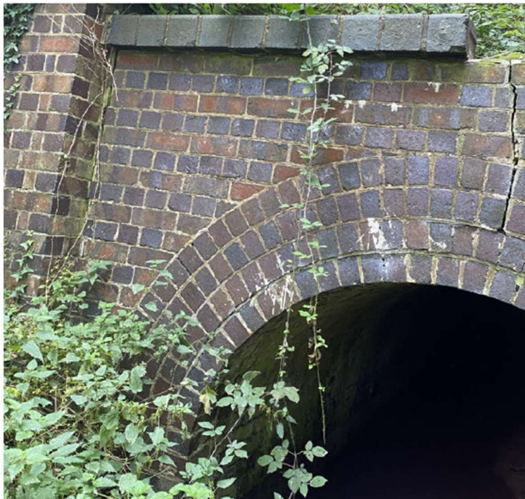
Figure 24: Crack through mortar joint at west end elevation of masonry arch barrel
