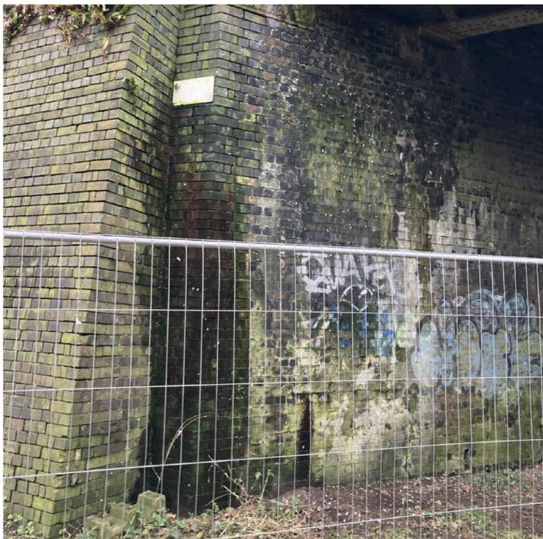
Figure 4-8 - Wet area on abutment wall
