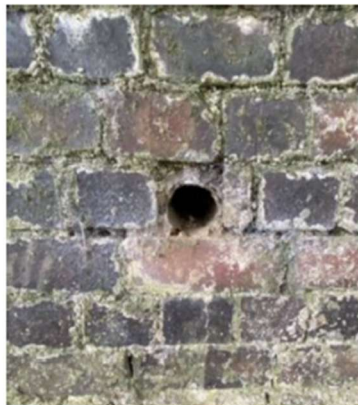
Figure 5.26: South abutment corroded drainage pipe
