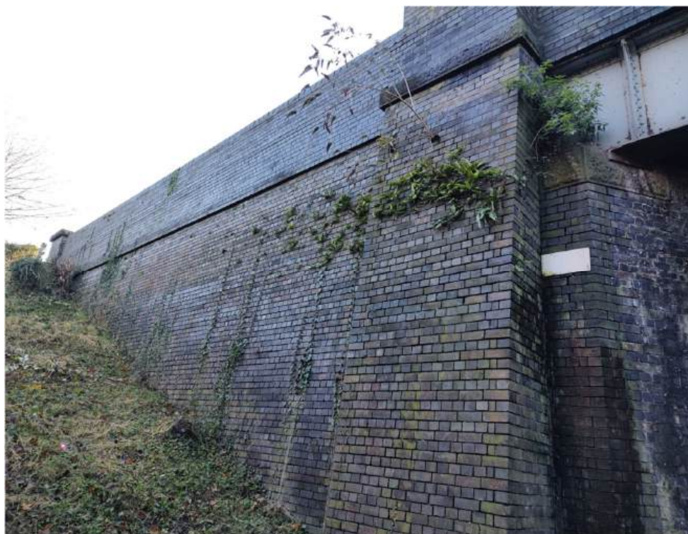
Figure 4-11 - Northeast wingwall vegetation in masonry
