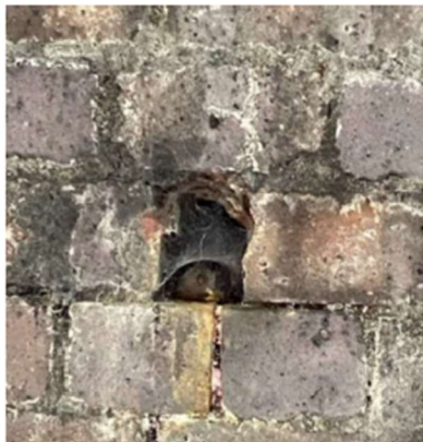
Figure 5.25: South span corroded drainage pipe
