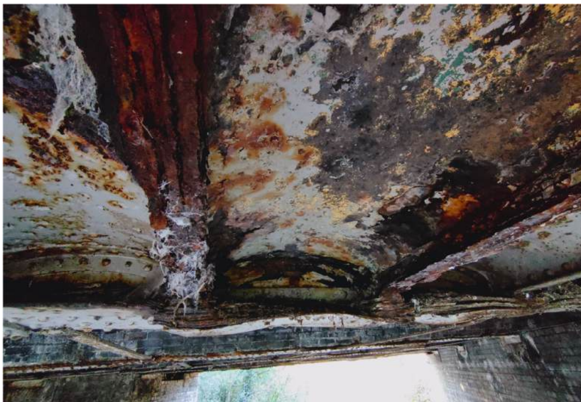
Figure 7-5 - Heavily corroded arches and flange deflection (NW)
