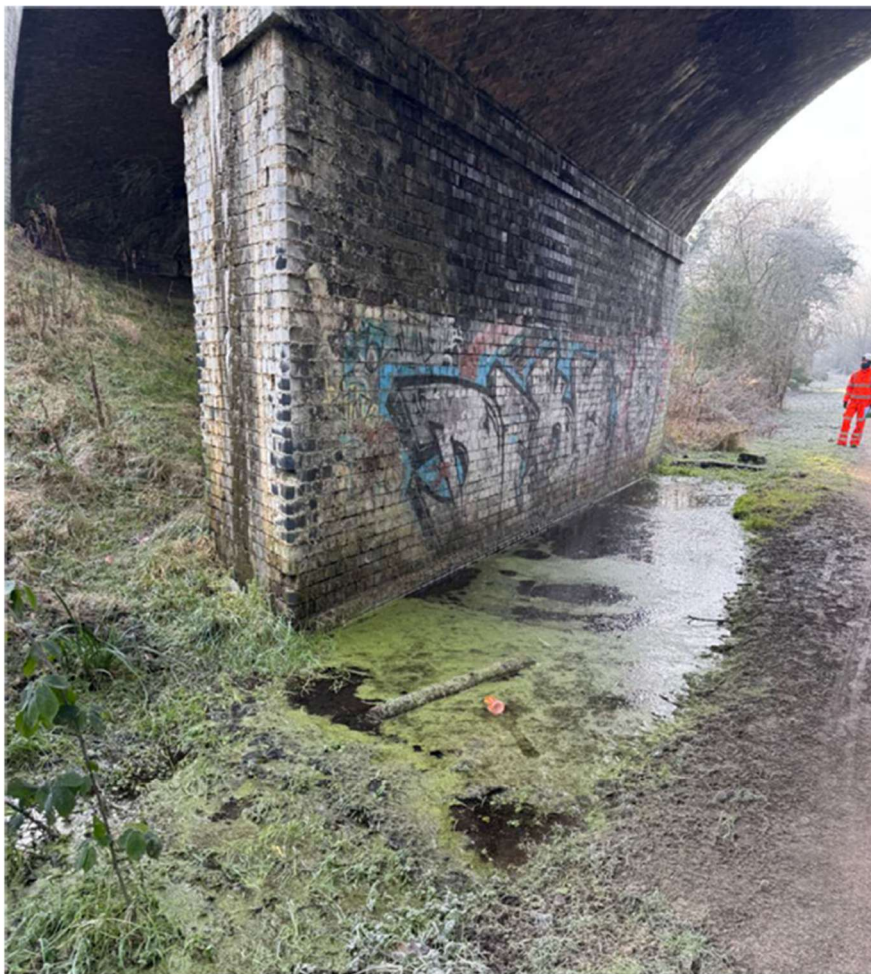
Figure 4-6 - Flooded base of pier
