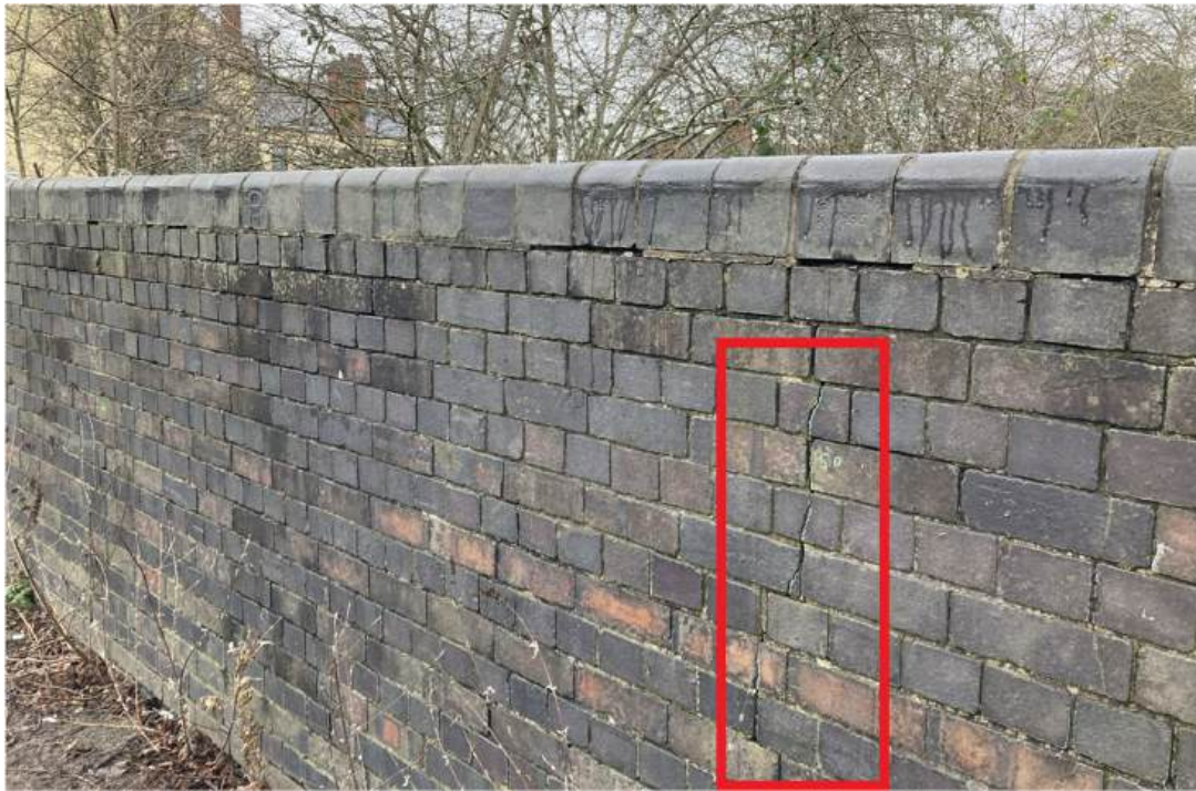
Figure 4-9 - North parapet with 5mm crack
