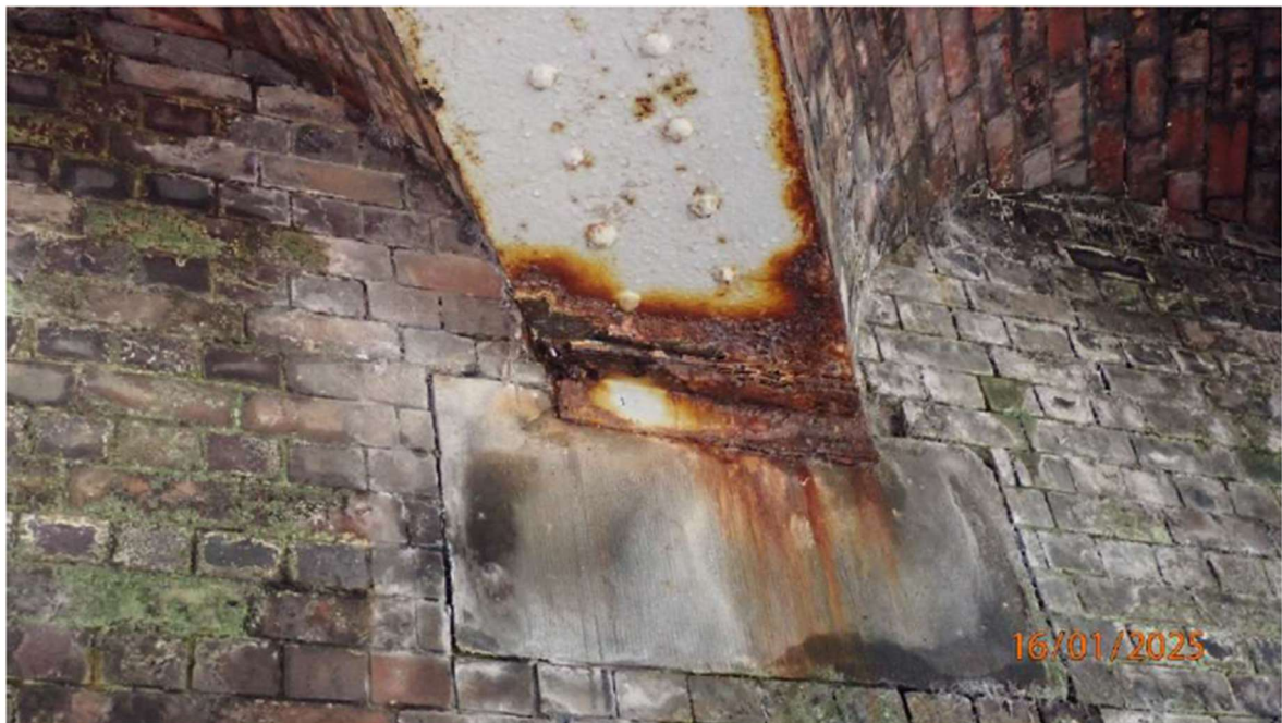
Figure 4-12 – Severe corrosion to the steel girder resting on padstone
