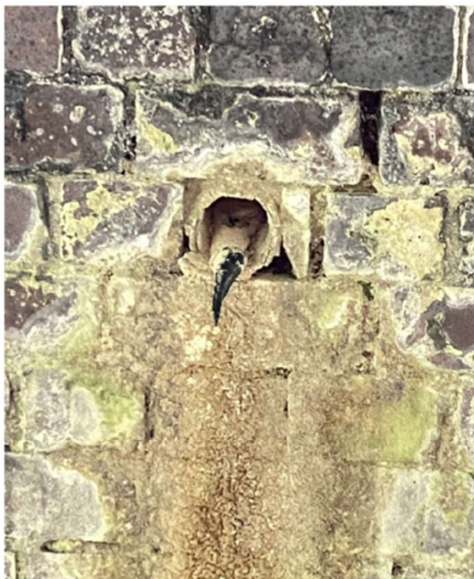
Figure 5.3: Blocked weep hole and associated water stains and mortar loss under arch soffit in Span 1
