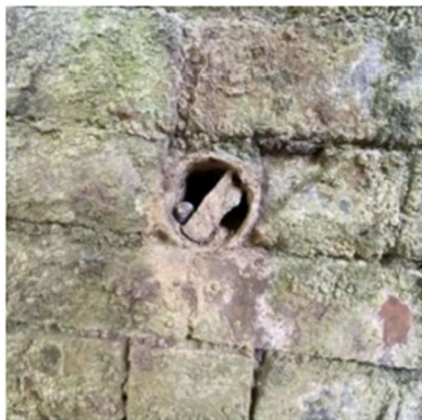
Figure 5.23: North abutment corroded and obstructed drainage pipe
