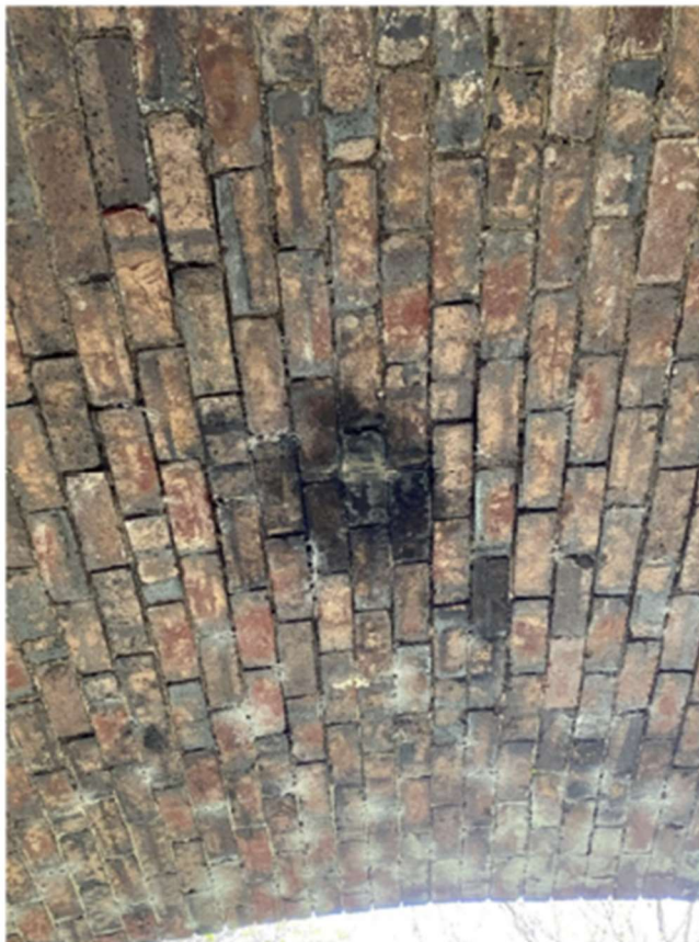
Figure 5.8: Seepage and signs of efflorescence under arch soffit in Span 2
