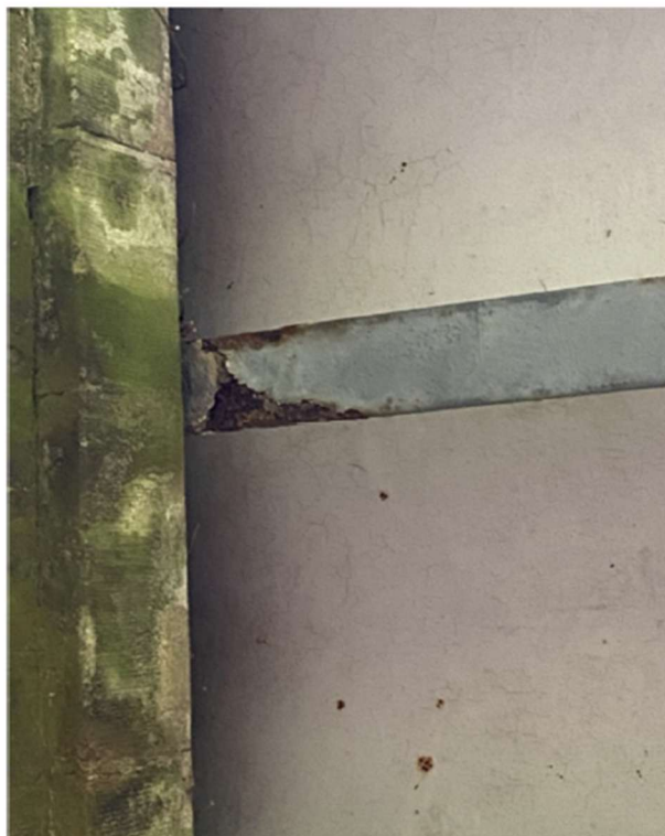
Figure 5.5: Concentrated corrosion to the main beams near the support location adjacent to the south abutment
