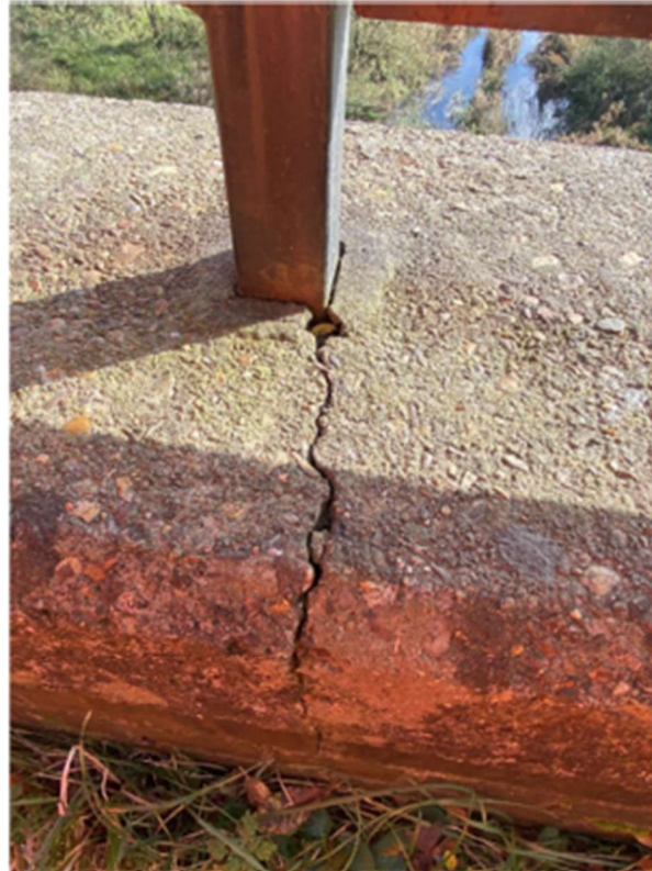
Figure 5.19: Cracking to the top of the east concrete parapet stringcourse at interface with parapet post
